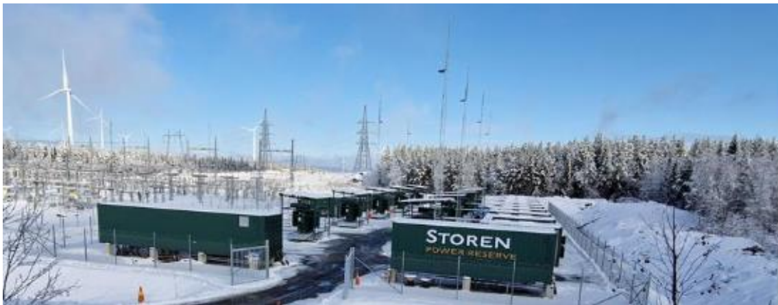
Battery Energy Storage Systems
